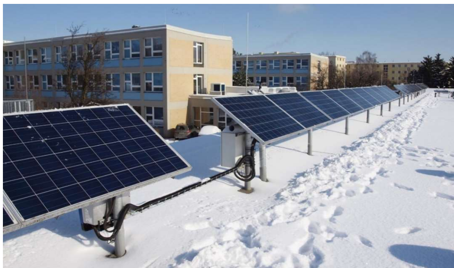
Fig. 1 On-grid PV system installed on the roof of the Faculty of Engineering in Prague
